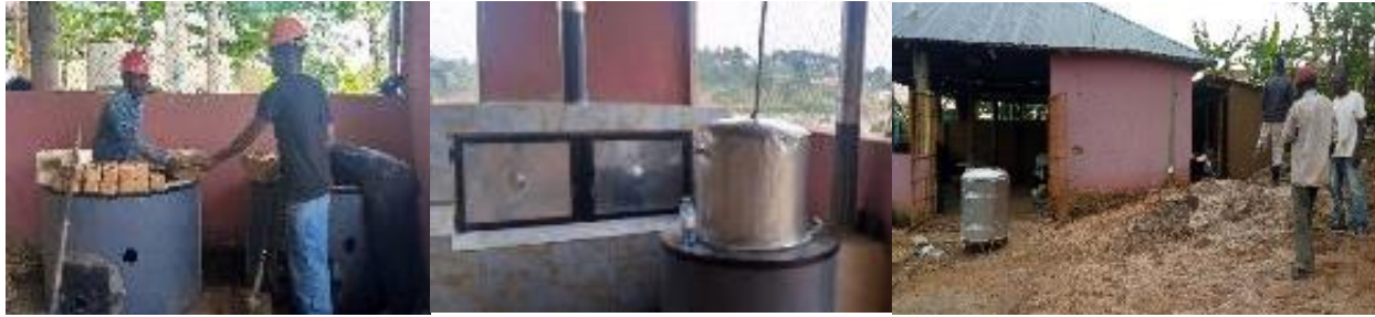
From left: construction of energy saving stove for frying, complete wood fuel oven with steamer in front and modification on bakery building on going
