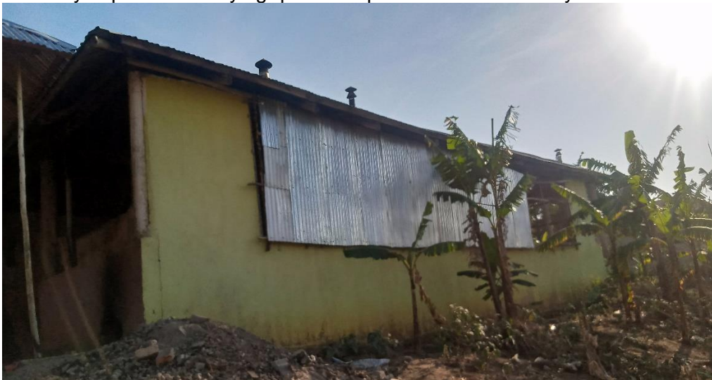
Formerly open spaces that have been closed with iron sheets to retain enough heat in the factory for proper doughnut expansion
