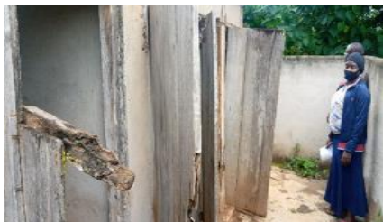
State of toilets Kitanda Primary school Gombe division Nansana Municipality Wakiso district
