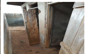
At Kiwala P/S, New doors need to be fixed, the old ones were found eaten up by termites, Floor needs to be cemented
