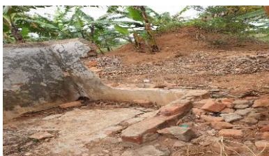
Girls' toilet at Butende primary school collapsed. Bathroom with a door needs to be reconstructed
