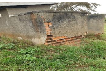
Washroom needs renovation. Cementing of the floor also needed
