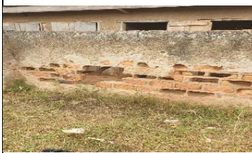
Butende P/S toilets need to be renovated for the dented walls, cementing the floor. 2 doors needed.
