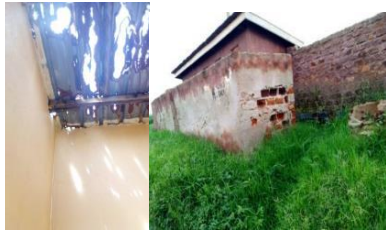
Replacement of iron sheets on toilet roof , work on the toilet walls and cement the floor at Lwadda Primary School
