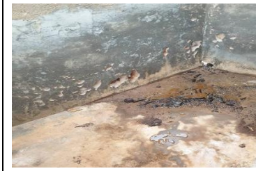
Butalunga P/S: Washroom floor needs renovation by cementing.
