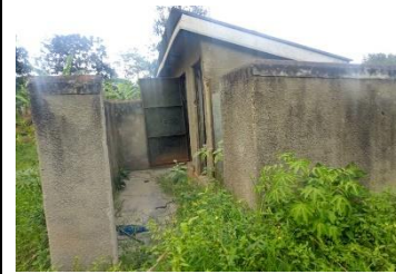
Floor needs cementing, doors need fixing (Butalunga P/S)
