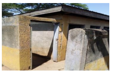
Fitting a door on a washroom and repair of the floor At Kitungwa Primary School
