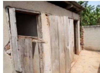
Three doors to be fitted at girls toilet and renovating the floor at Kitanda Church of Uganda Primary School
