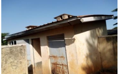
Fitting gutters on toilets to supply water to the tank and fixing two taps
