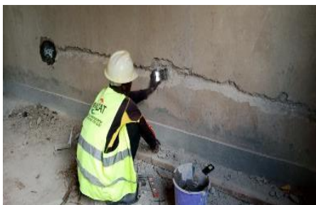
The happy pad promotion centre being fitted with electricity and enough sockets and switched at Katalamwa Secondary School in Wakiso district
