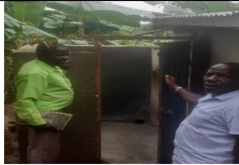
<After> The washroom was fixed in terms of its location and the door well fixed with a lock
