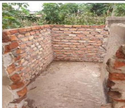
<After> The toilet block which was being used as a washroom but a new washroom and a changing room under construction
