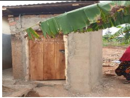
<After> The school did not have a changing room which was improvised, fixed a door and roof and plastered
