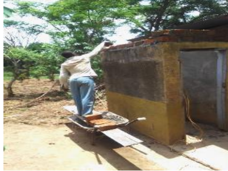
<After> The girl's wash room had no door and the floor was rough so the school resolved to fix a door and work on the floor and the walls.
