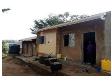
<After> Tank had no gutters supplying water. Gutters fixed and water flows into the tank when it rains fixed
