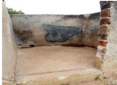
a hole on the wall which was filled up and covered.
