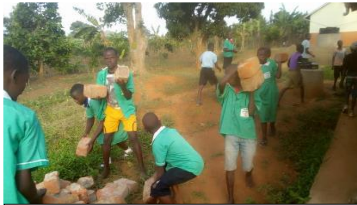
Lwamasaka P/S Boys involved in the renovation of girl's washroom/changing room in Butambala district
