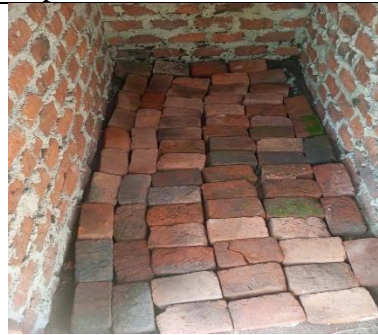
Inside part of the changing room at Kiyita P/S
