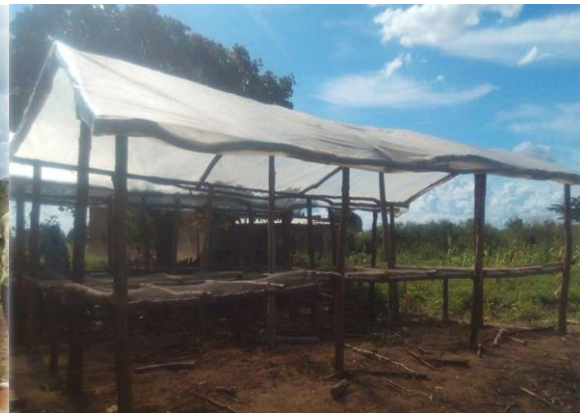
Drier shade with solar drier tarpaulin
